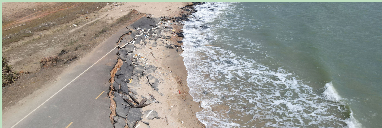
The road in southern Thailand eroded by rising sea levels.
