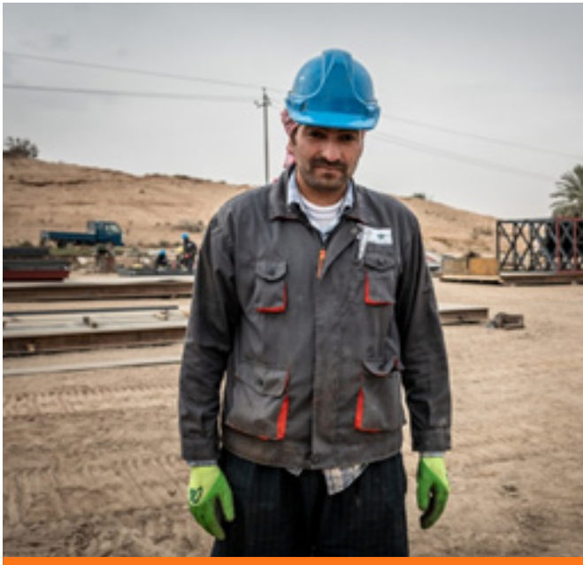
Salah, 38, Construction worker repairing Al Khoor bridge, Qaim. Rehabilitation of the bridge was completed by FFS.
